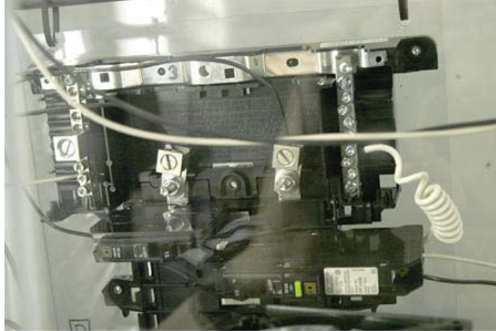
Figure 5. Photograph of load center circuit.
